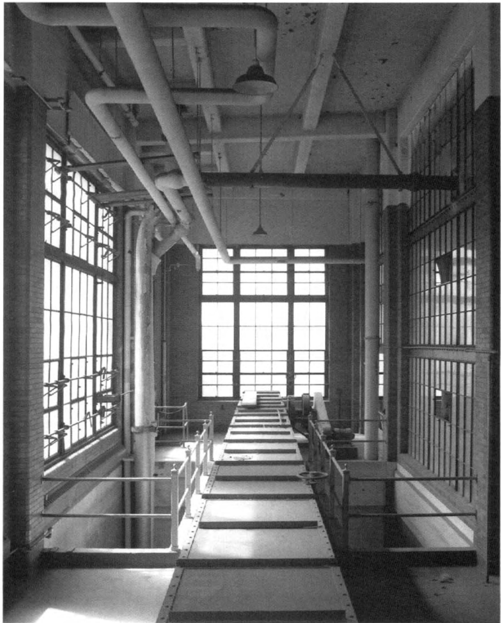
STEAM PLANT, FORD MOTOR COMPANY, ST. PAUL, 1992
